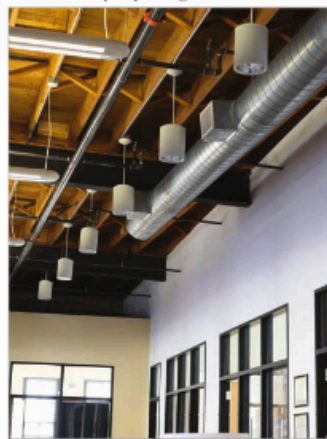
Before – CFL downlights, mostly burned out, ready for LED retrofit
